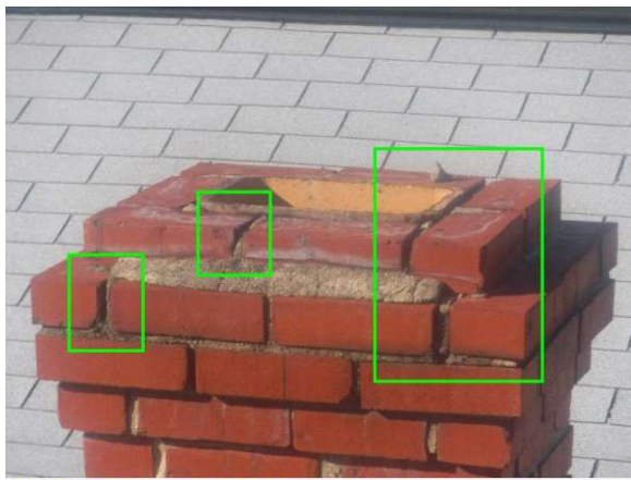
Missing / damaged mortar on chimney cap
