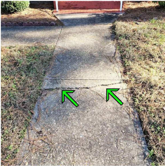
Minor uplifting in front walkway
