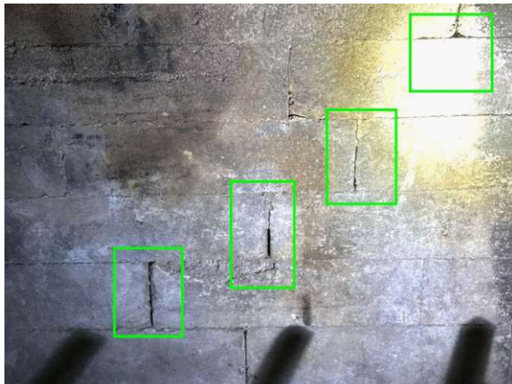
Cracked / missing mortar in firebox
