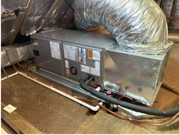
Air handler in attic
