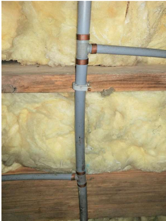
Polybutylene (PB) piping in crawlspace
