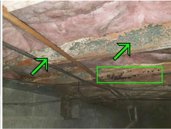
Organic growth on floor joists
