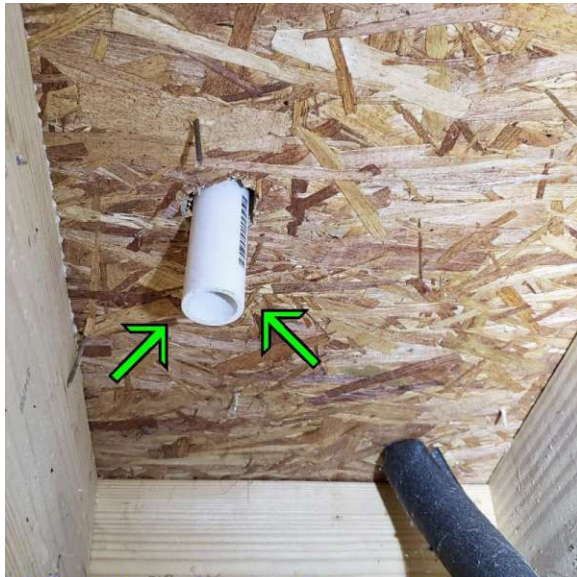
TPR discharge pipe routed to crawlspace
