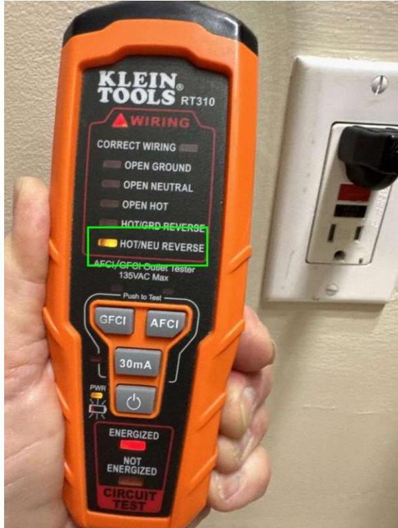
Improper wiring - Hot / neutral reverse
