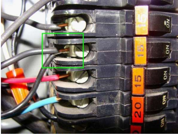
Double-tapped 15-amp breaker
