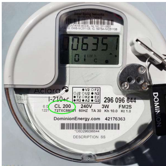
200 amp service meter
