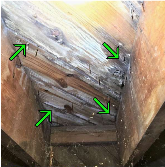
Subfloor damage / Right rear
