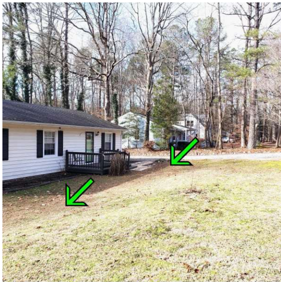
Front yard slopes towards house
