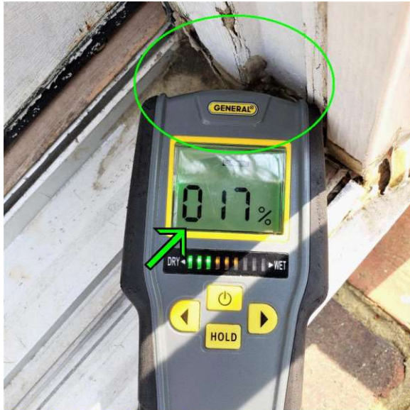
Wood rot / High moisture content
