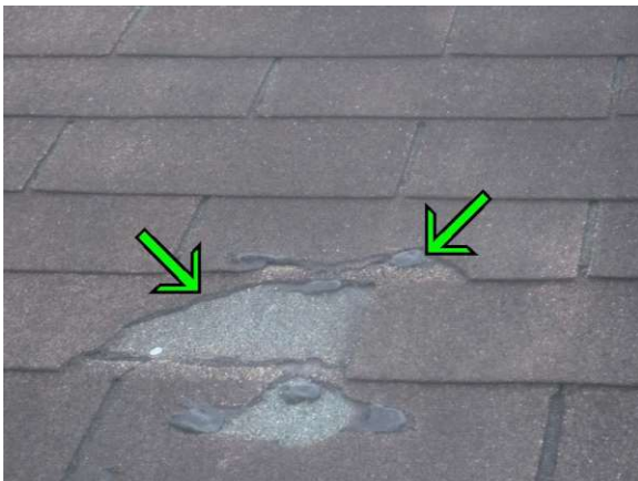
Shingle damage / Right front
