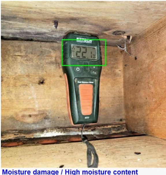
Moisture damage / High moisture content
