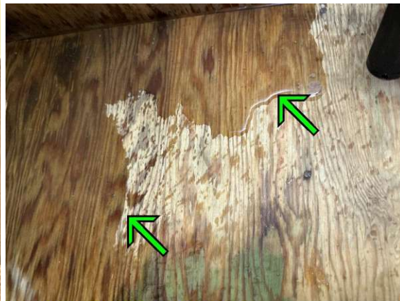
Area under waste / drain piping
