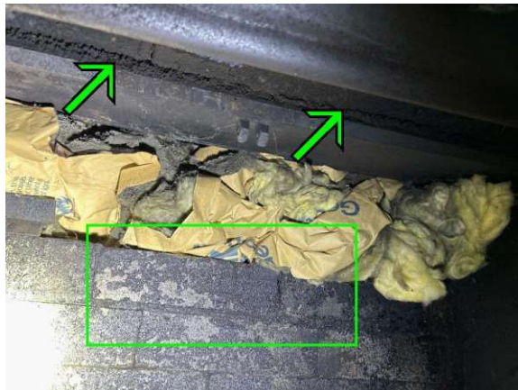
Creosote build-up at damper
