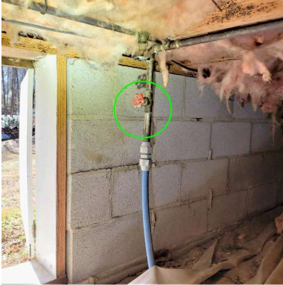
Main water shutoff
