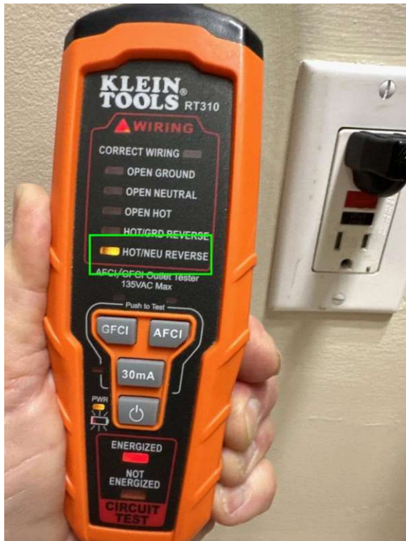
Improper wiring - Hot / neutral reverse
