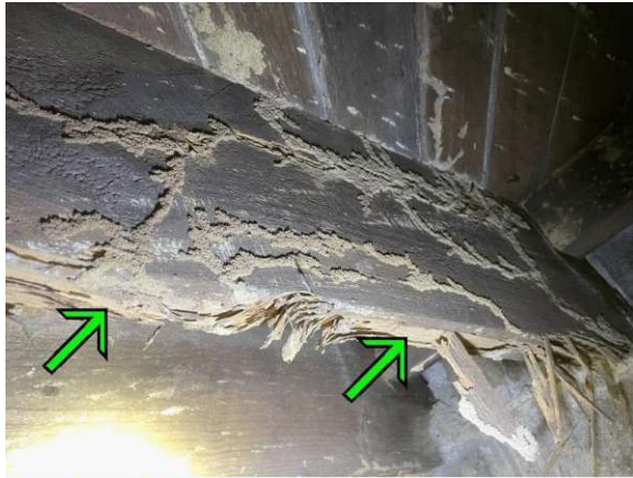
Possible WDO damage to floor joist
